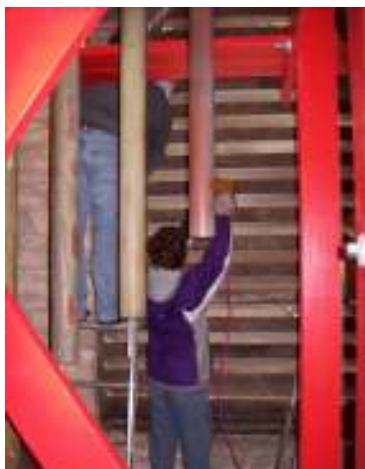
Letting the sound out. Here is a photo of Sean Weston & Dan Clark installing screen on the louvers on the east side of the chime loft. The louvers had been sealed with metal for many years. December 20 th
